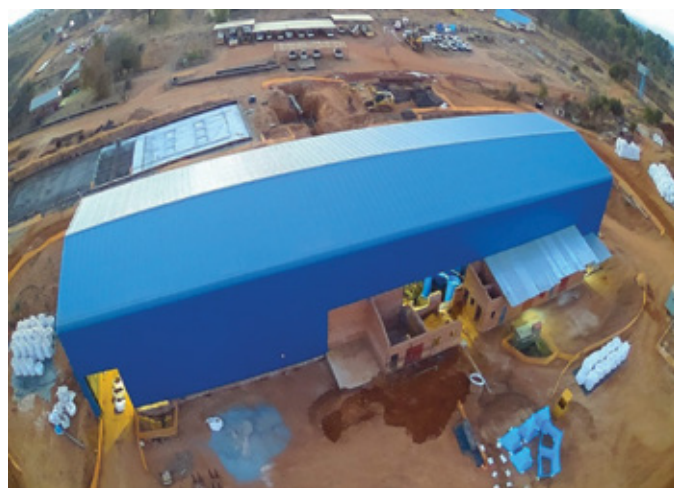
FIGURE 2: June 2025: 50 MLD up and running
