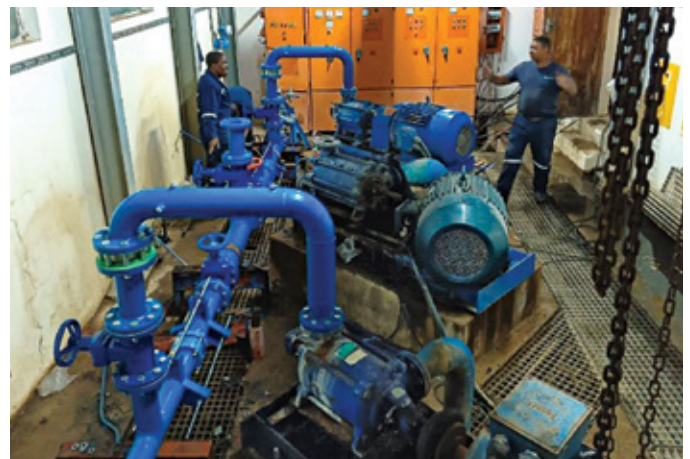
FIGURE 4: MCC and new pipework in service (after)
