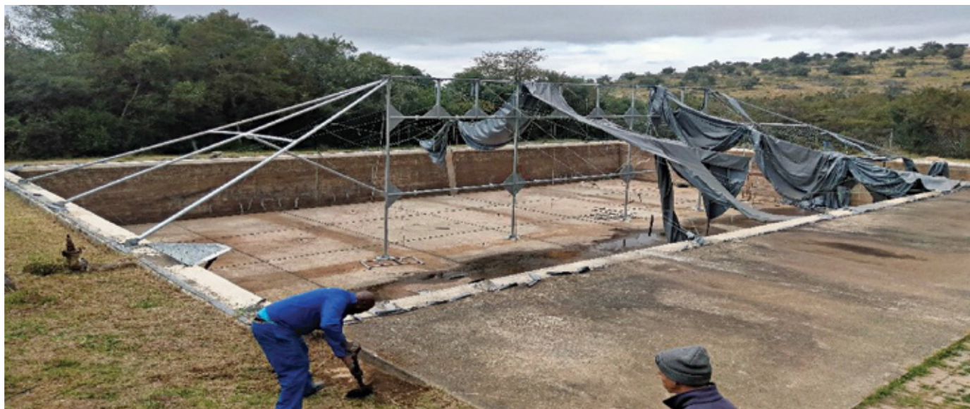
FIGURE 5: Damaged Potable Water Storage Reservoir (before)
