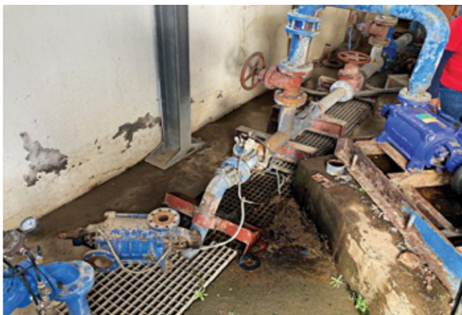
FIGURE 3: Suction pipework in advanced state of corrosion (before)
