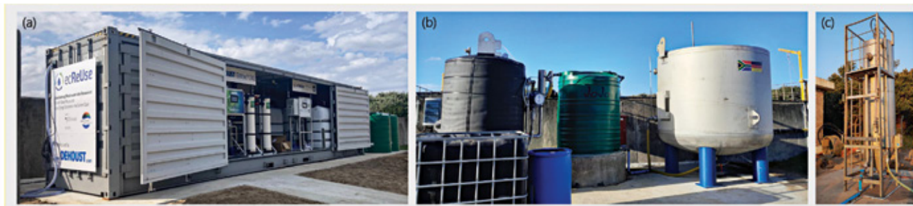
FIGURE 4: Pilot units installed at the East Bank WWTP: (a) MBR system, (b) primary sedimentation and anaerobic reactor, (c) continuous sand filter.
