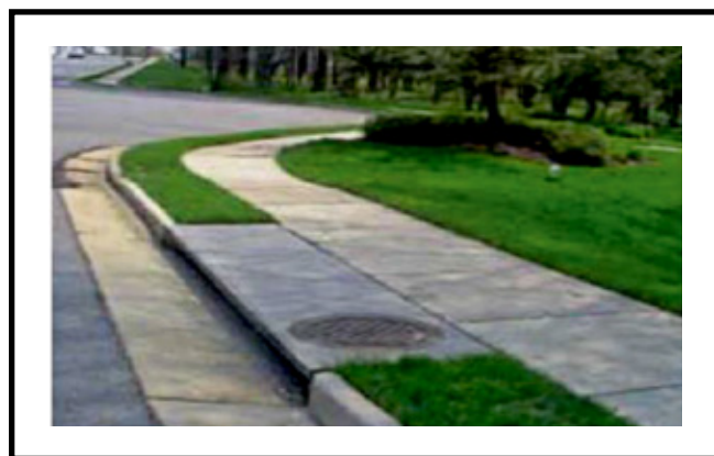
FIGURE 12: Existing kerb inlets without transition
