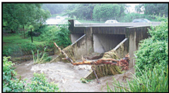
FIGURE 8: Typical example of debris fins
