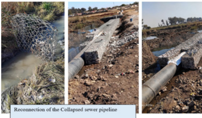
FIGURE 7: Showing newly constructed sewer line protected by gabions to prevent future damage
