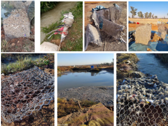
FIGURE 6: Showing waste water screens installed within the channel to trap solids before reaching the river
