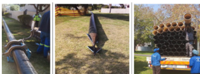
FIGURE 9: Showing Engineering intervention (trenchless technology)- Pipe cracking material and HDPE Welding system
