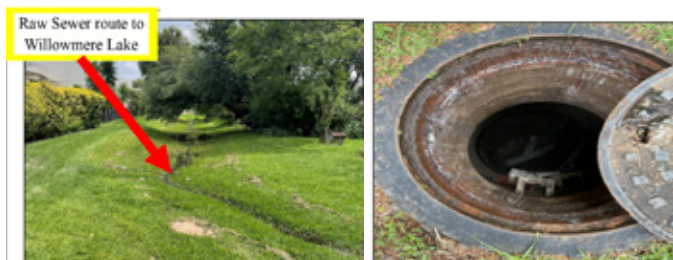
FIGURE 7: Showing channel where raw sewer flows into the Willowmere Lake
