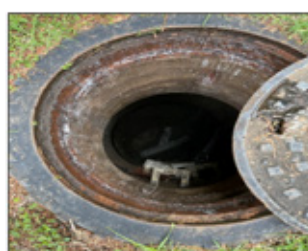
FIGURE 8: Showing sewer manhole where raw sewer overflow to the Willowmere Lake
