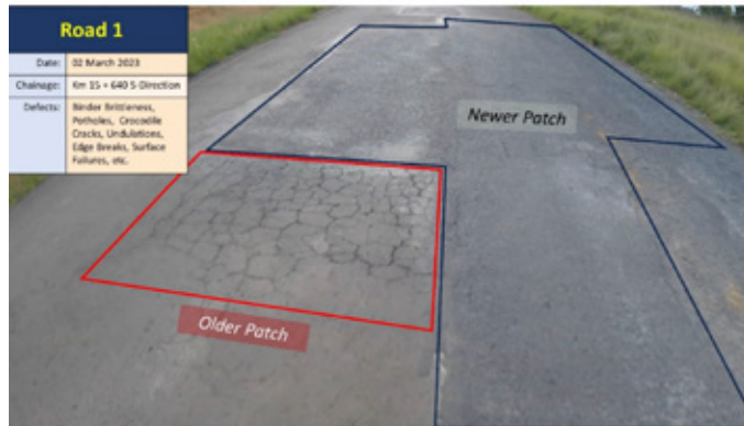
FIGURE 3: Road 1, Older patch indicating poor performance.
