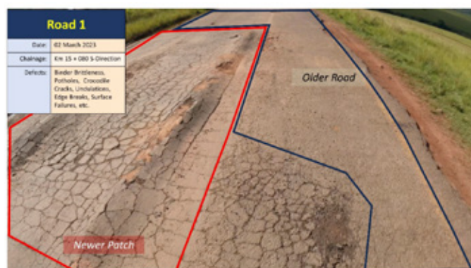
FIGURE 2: Road 1, Patch performing worse than adjacent older road
