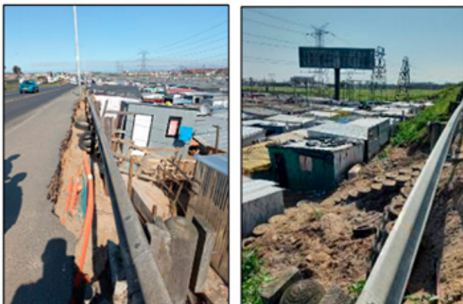
FIGURE 7 & FIGURE 8: Encroachment onto fill embankment
