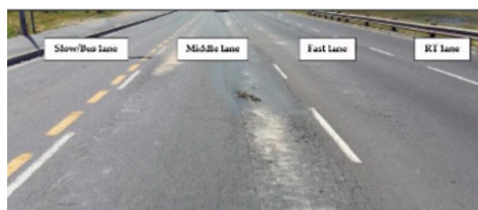
FIGURE 4: Crocodile cracking and pumping on northbound lane
