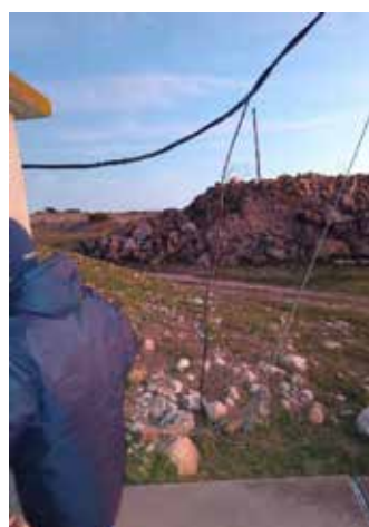
FIGURE 9: Attempted cable theft causes water disruption
