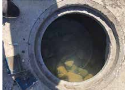
FIGURE 6: Malicious vandalism – rock filled chamber
