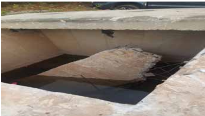
FIGURE 11: Unbraced cover slab collapse due to an intrusion attempt
