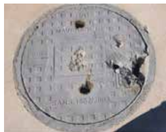
FIGURE 17: Polymer concrete lid after vandalism
