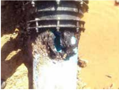
FIGURE 5: Vandalism by arson
