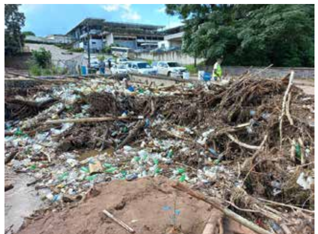
FIGURE 7: Caversham Culvert blockage
