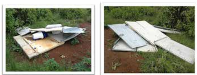
FIGURES 9(A) AND 9(B): Failed Structures with no Certification in Eastern Cape
