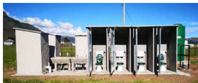
FIGURE 10: Low Flush Toilet Facilities installed in Schools in Eastern Cape
