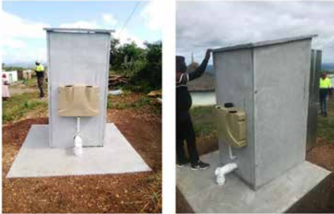
FIGURE 12(A) AND 12(B): Individual Household Units installed in the Eastern Cape with rear mounted Demand Flush Tank and leach pit directly below
