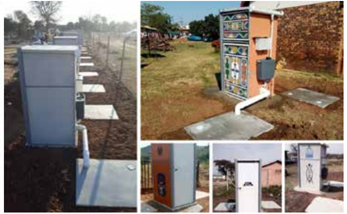
FIGURE 13(A), 13(B), 13(C), 13(D) AND 13(E): Sanitation units with off-set dual leach pits with rain water harvesting and externally mounted demand flush tank
