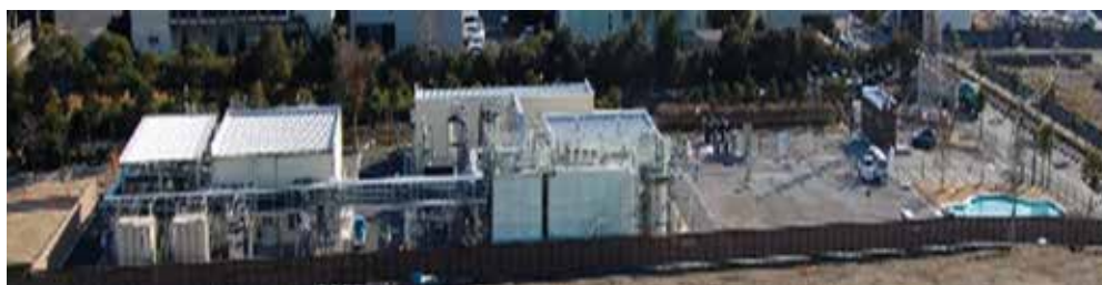
FIGURE 4: Kita Kyushu Remix Water Plant (Source: Hitachi Ltd.)
