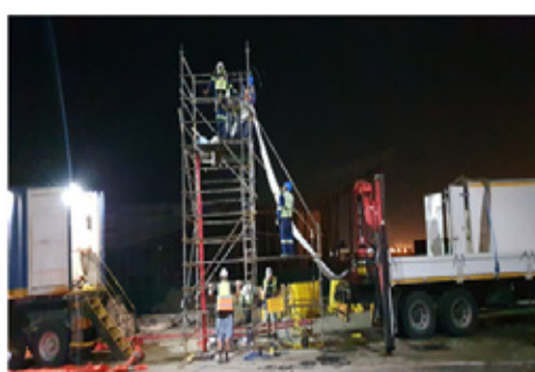
FIGURE 32: CIPP liner being installed by the inversion process cured by hot water using a boiler
