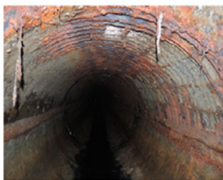
FIGURE 1: Corrosion inside existing 1350mm diameter concrete pipe
