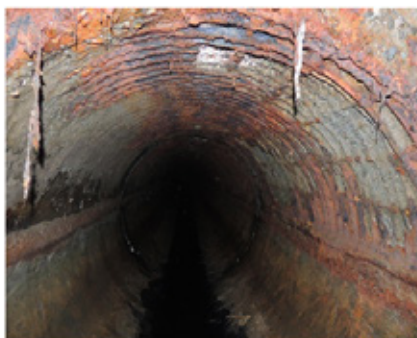
FIGURE 25: 1350mm diameter pipe before rehabilitation
