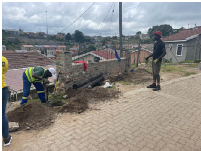
FIGURE 1: Concordia Road Phase 1 - EME's digging holes for the erection of Guardrails posts.
