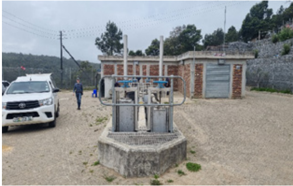
FIGURE 1: Thembalethu Pump Station
