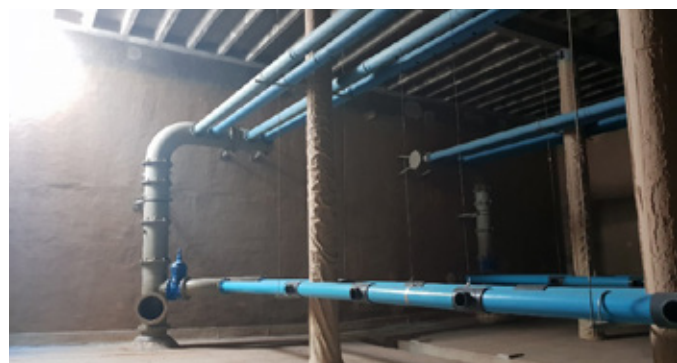
FIGURE 11: Launders inside the reservoir to collect settled water
