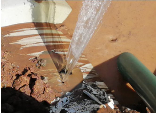
FIGURE 2: Loss of pipe material due to corrosion (Rand Water Photographs)
