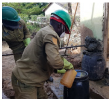
FIGURE 5: Often the only practical way to empty pit latrines is manually. The use of suitable personal protective equipment and long handled tools makes the job less unpleasant and less hazardous.
